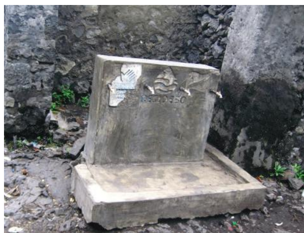
Figure 19: Community water point in need of repair
